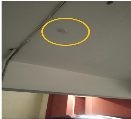
Figure 4. Beacon in the parking lot
